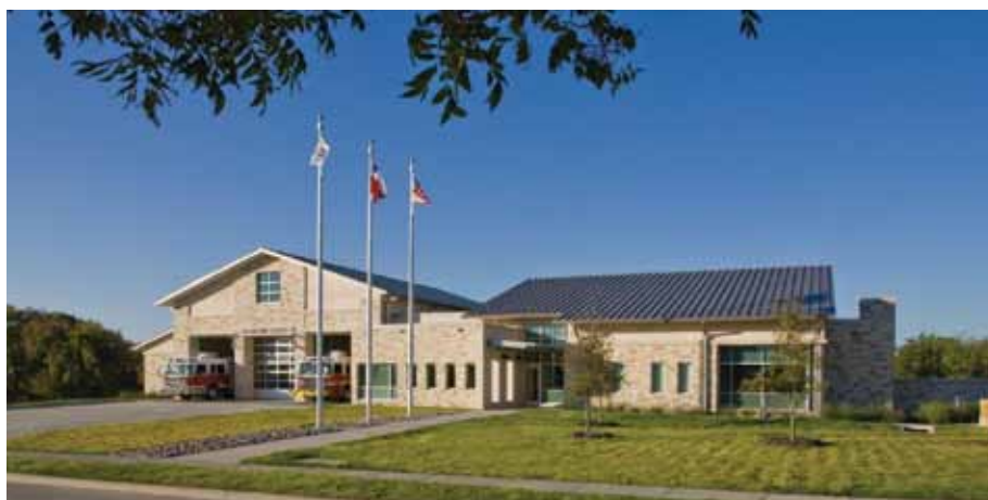
The 15-ton heat pump installed at Plano (TX) Fire Station No. 13 offers the opportunity to test the operating costs of gas vs. electric cooling. Energy use and cost at the station will be compared with that of another "twin" station using electric cooling technology.
