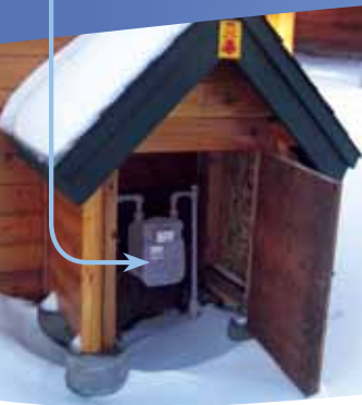
■ Meter with snow shelter
