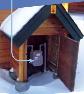
■ Meter with snow shelter
