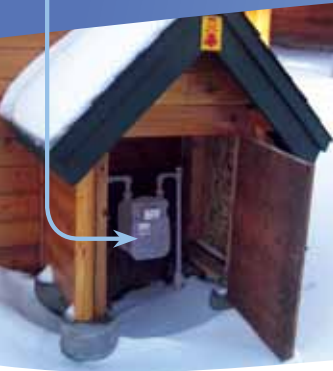
■ Meter with snow shelter
