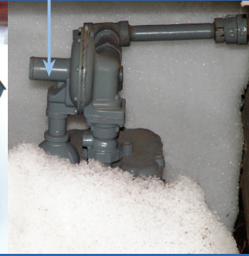
■ Meter without snow shelter
