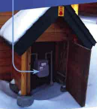
■ Meter with snow shelter
