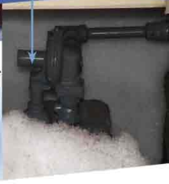
■ Meter without snow shelter
