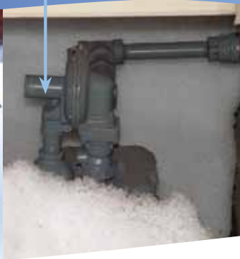
■ Meter without snow shelter
